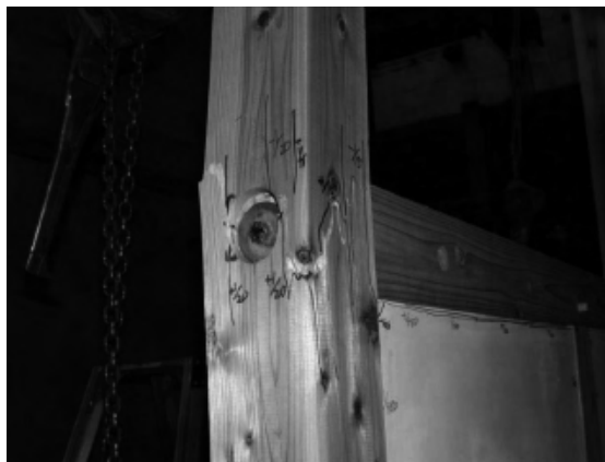
(c) 窓台部中柱曲げ破壊
