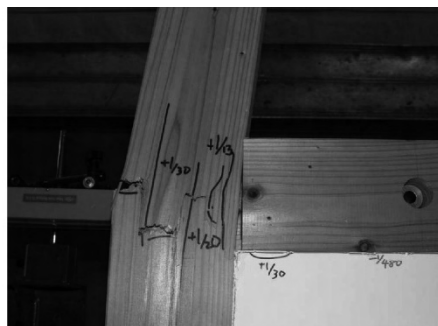
(c)窓台部中柱曲げ破壊
