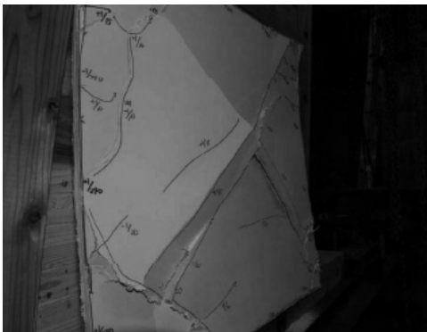
(b) 腰壁の漆喰のひび割れ
